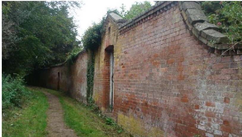
Picture 15. A fine brick wall important and visually prominent in the public domain adjacent to a well used footpath. As can be seen some repairs necessary and consideration should be given to the removal of selected vegetation.
