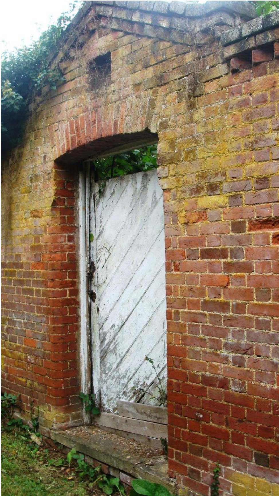
Picture 26. Wall and door adjacent to footpath 16 would benefit from repairs.
